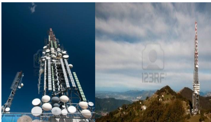
Figure 4. Big television and radio tower with several parabolic antenna on high quote (mountain) - Roncola (Italy)( http://www.123rf.com/photo_10872365_big-television-and-radio-tower-with-several-parabolic-antenna-on-high-quote-mountain--roncola-italy.html )
